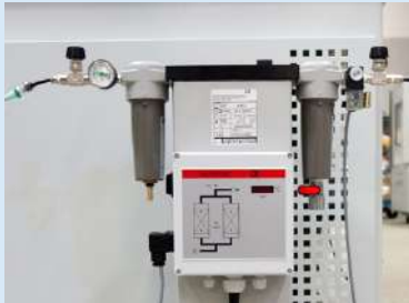
Additional Drying Capacity
